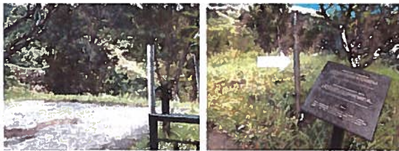
Sella Bay Safety hazards, lack of railing structures, protruding poles, vandalized signage
