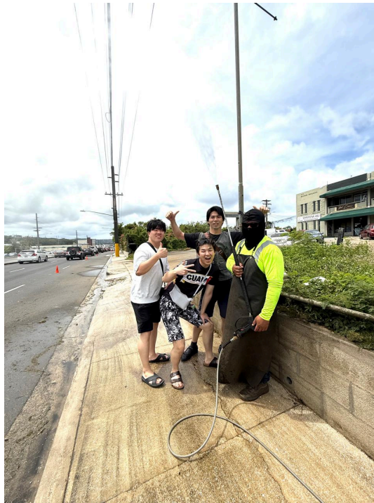
GVB maintenance teams waterblast a retaining wall along Marine Drive, while visitors stopped to say, "Oh Yeah!"
